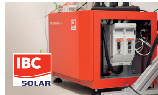
IBC SolStore 6.5 Li / IBC Solar
